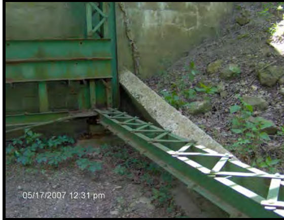
West corner wall leaning.
