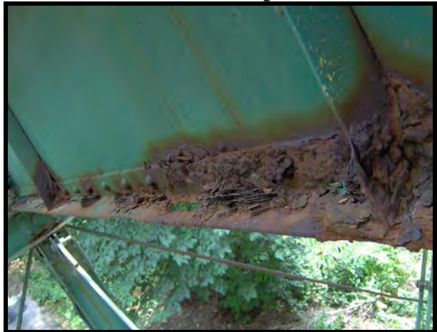
FB #2 6 L 9 (W) of (E) truss 1½' x 7" hole rusted through bottom outstanding angle leg to (N) Span #4.
