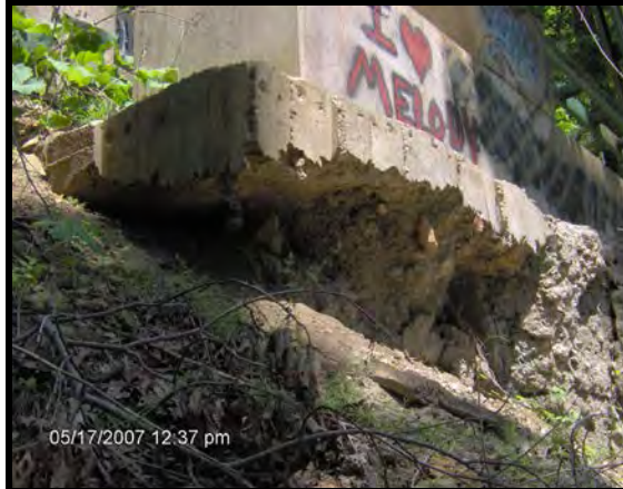
Third Pier void under west side of Pier Cap.
