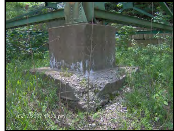
First Pier spalled pier caps.
