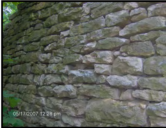
South Abutment stones falling out.
