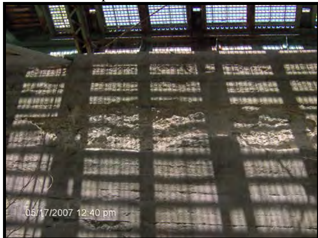
North Abutment spalding.
