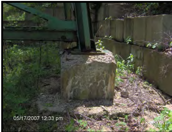
First Pier spalled pier caps.
